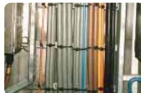
Marine Cable Bundling
