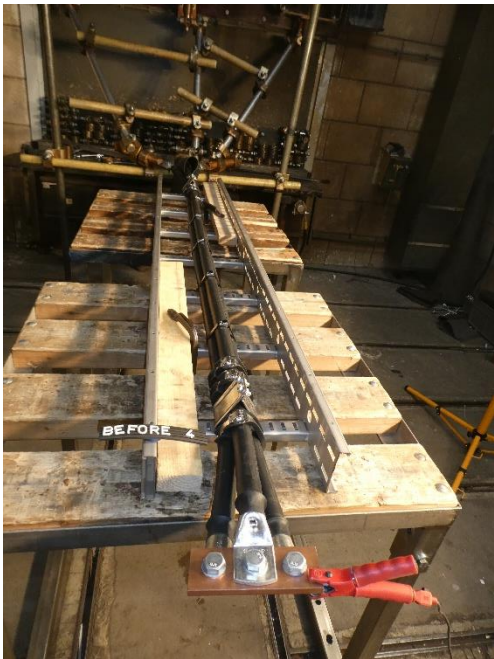
Photo 1 Cable cleats for electrical installations Manufacturer: Band-it IDEX Configuration: 5
